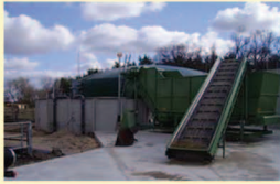
Biogas plant Schwechten (Germany)
